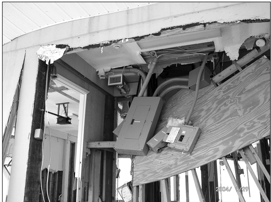
Figure 6. Non-compliant utilities attached to breakaway wall
