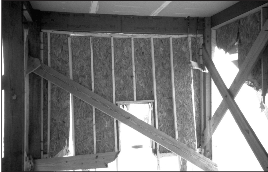
Figure 7. Non-compliant bracing arrangement
