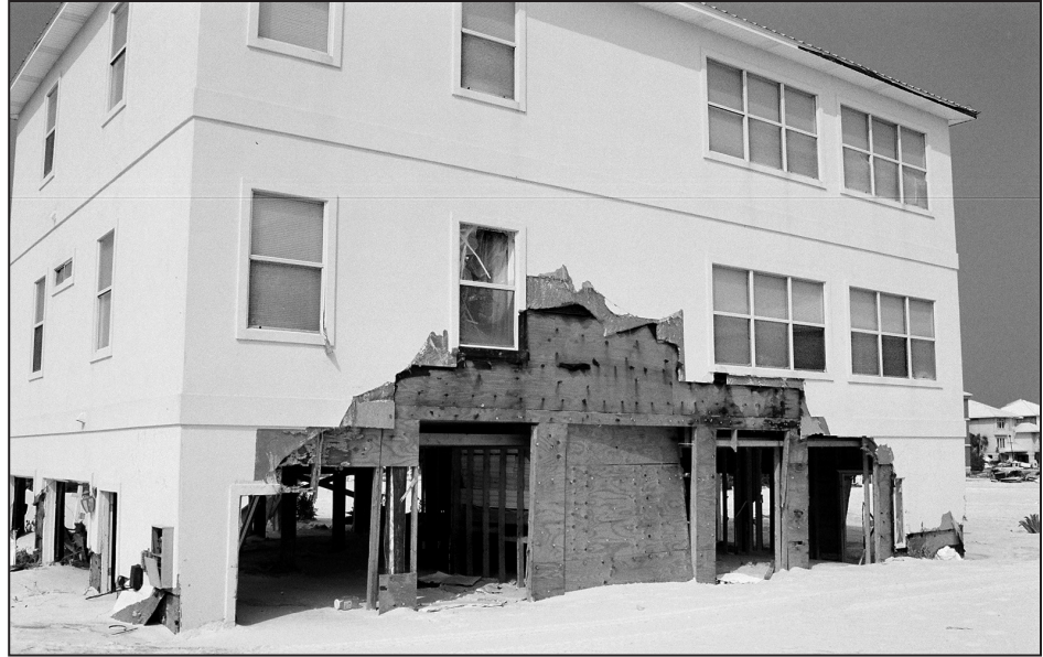
Figure 5. Non-compliant breakaway wall joint detailing
