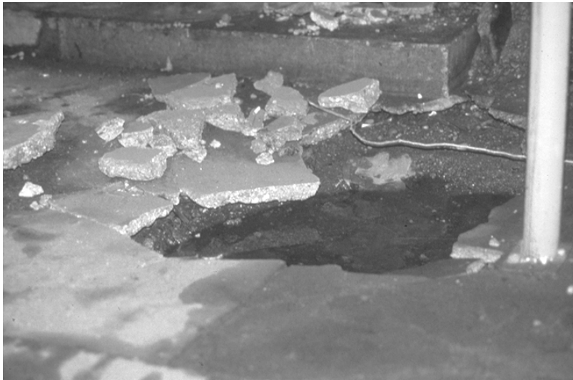
Figure 1-2. This basement floor broke from hydrostatic pressure
