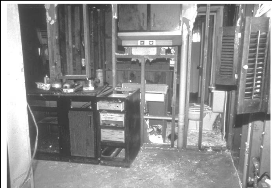
Figure 9-15. Even slow-moving floodwaters can cause substantial damage
