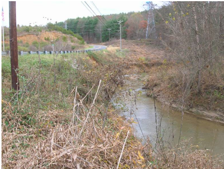
Looking upstream at the eroding stretch of bank.
