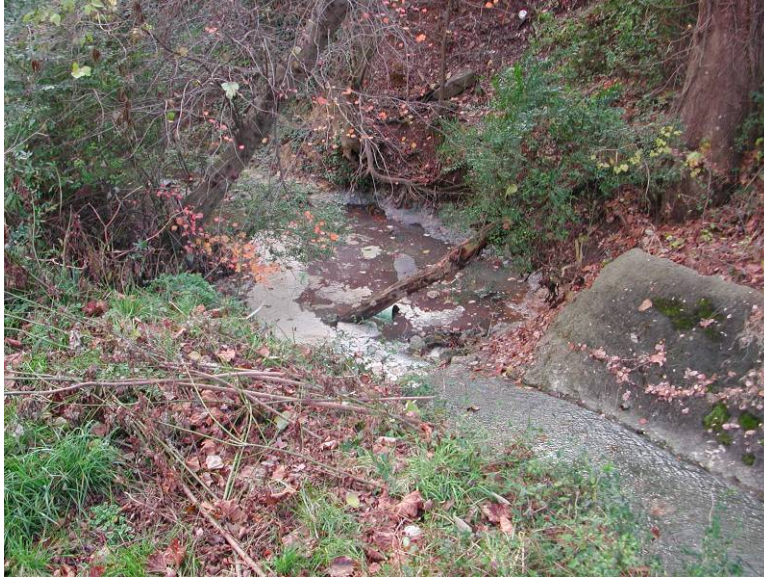
The bed of UT to Cub Creek has scoured significantly below the concrete channel. Water sampling here shows high concentrations of BOD 5 .
