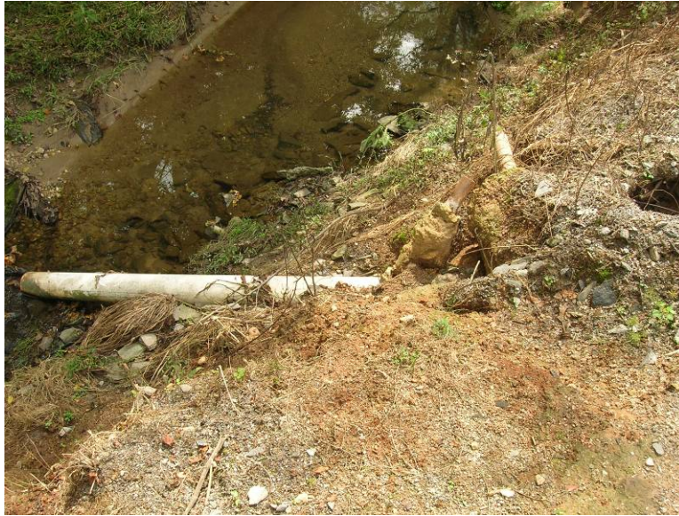
There are numerous outfalls into the channel along this reach of UT to Cub Creek.
